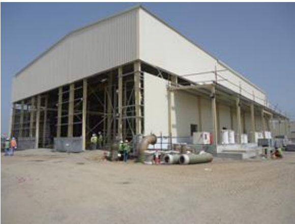
Figure 5 Barka Dissalination Plant Image
