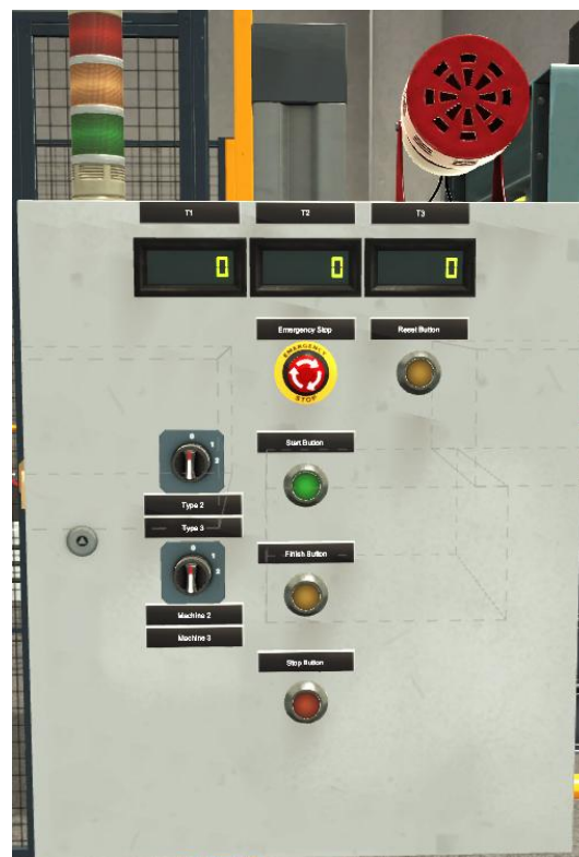
Figura 3-13. Panel de control
